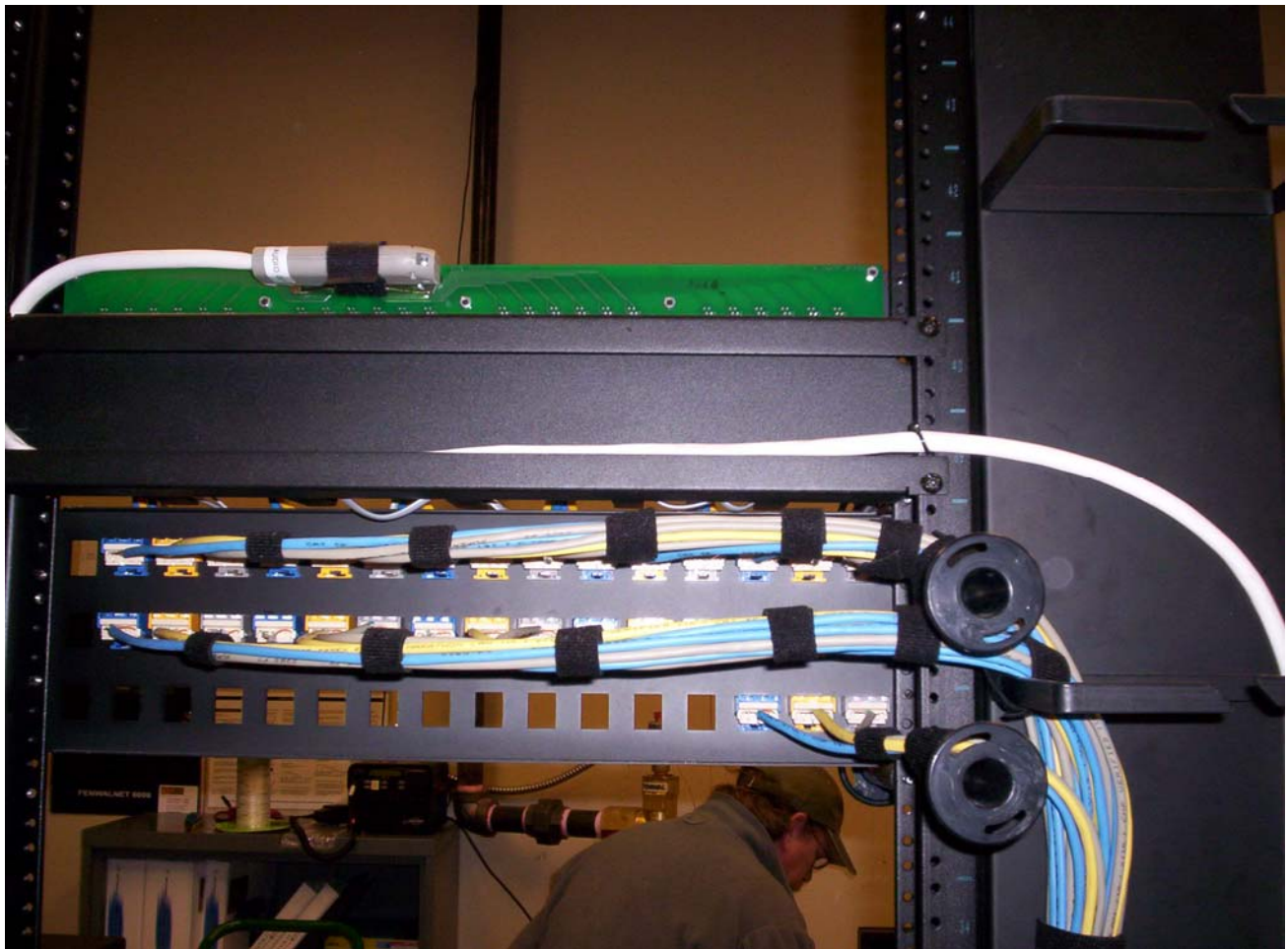
Figure 7-12: Example of Properly-Installed MDF Patch Panel Assembly
