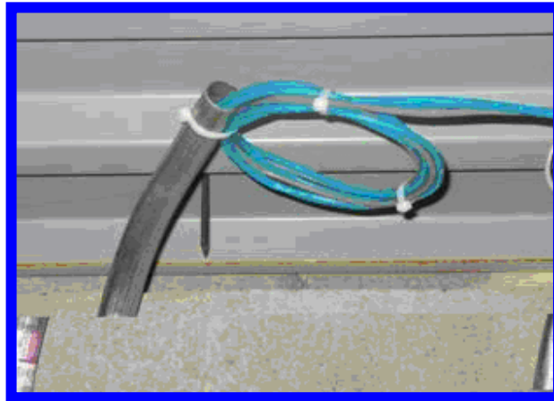
Figure 7-8: Example of Workstation Service Loop
