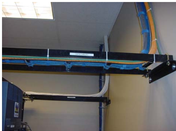
Figure 7-1: Example Wall-Mounted Ladder-Type Cable Rack
