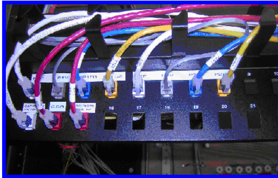
Figure 7-10: Example of an RJ45 Unloaded Patch Panel with Jacks (2 of 2)
